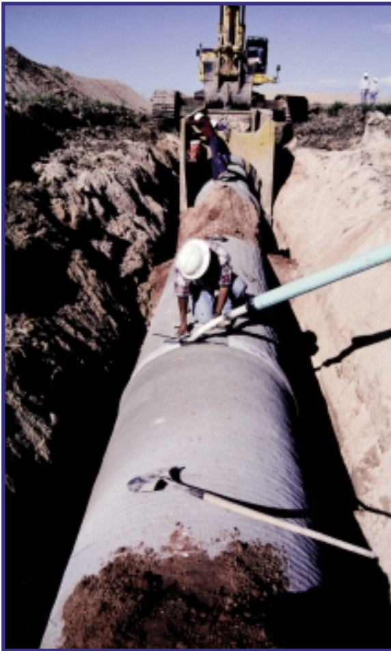
The joints are bonded and filled with grout immediately following the pipe laying operation.
