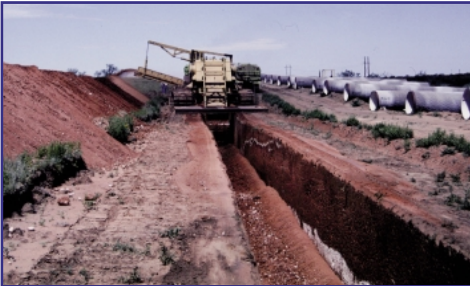
Jetco Trencher can open an 8 foot trench in sand, clay or solid rock.
