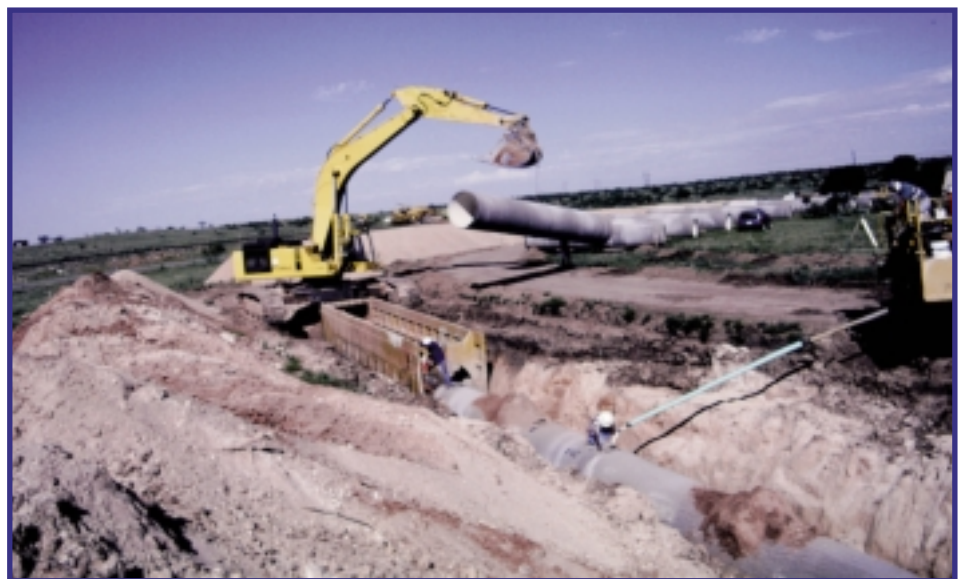
Installation contractor, J.D. Stephens, installed 189,000 feet of AWWA C303 Bar-Wrapped Concrete Cylinder Pipe in the Roberts County Project.
