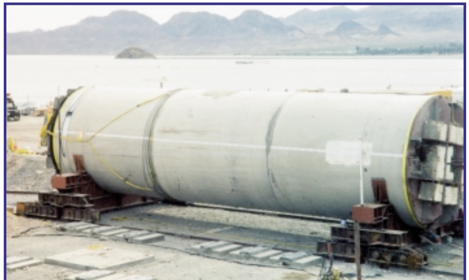
Triple 144-inch RCCP assembly weighing 180 tons with two temporary bulkheads in the launch way saddles on rails. The assembly is ready to be launched into the water.
