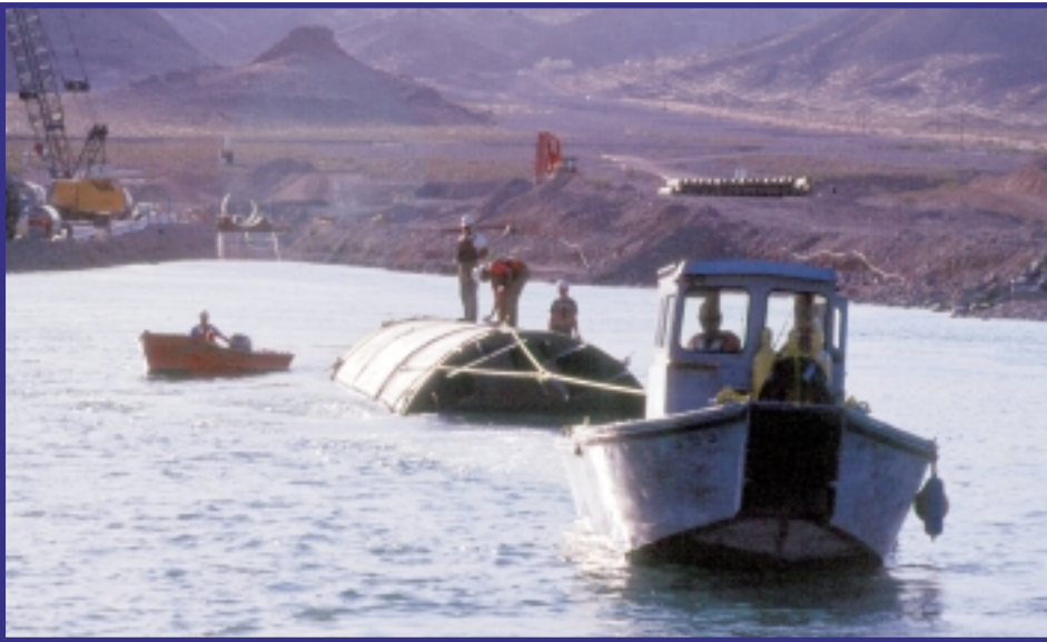
The floating assembly was pulled by a tug from the launching site up to the laying barge.
