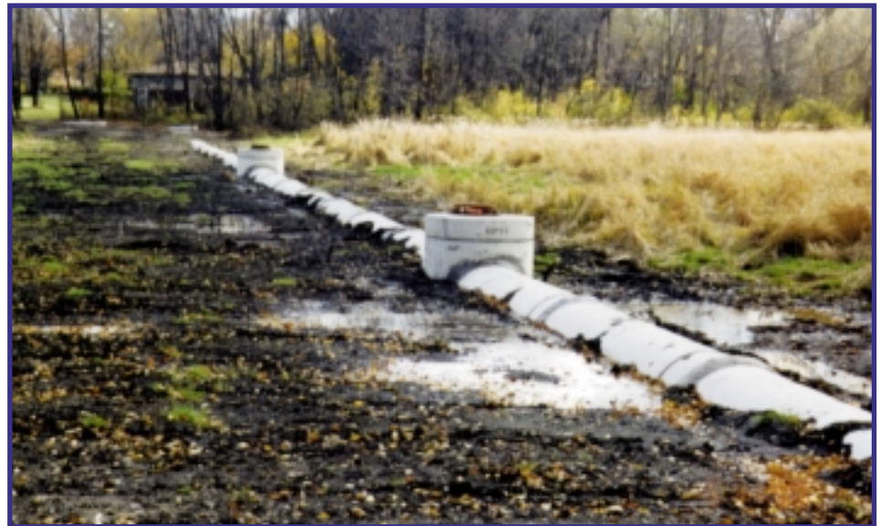
Crossing Patton Cemetery, PCCP was precisely placed on piles. Being acid resistant and immune to atmosphere exposure, PCCP was a natural choice for the project.
